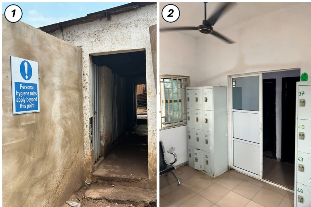
FIGURE 9. Typical washroom amenities as observed in ULAB recycling plants in sub-Saharan Africa
